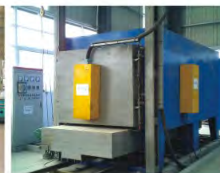
大型热处理设备 Large-scale Heat Treatment Equipment
